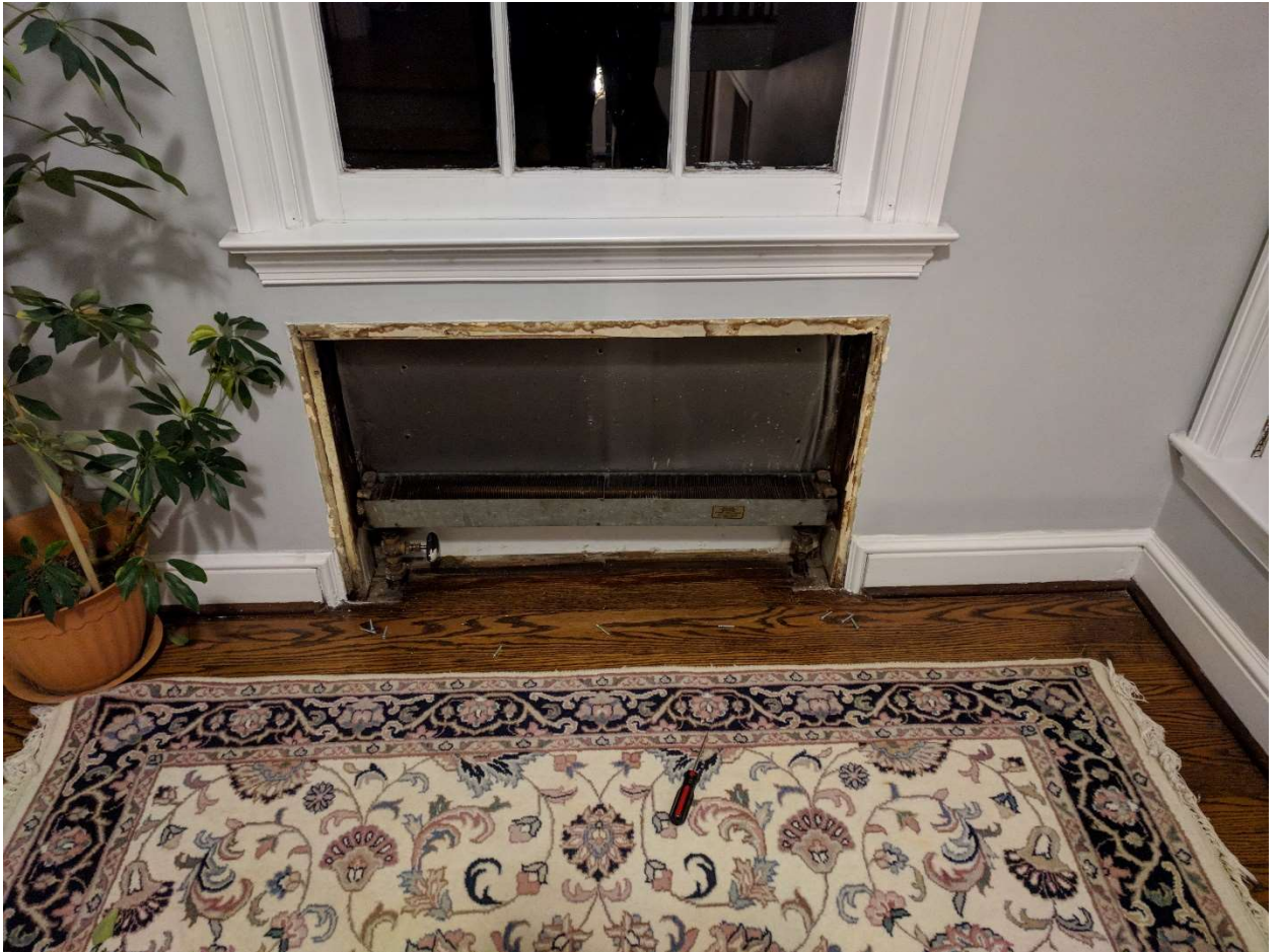
Center hall convector that bangs and has a plugged port
