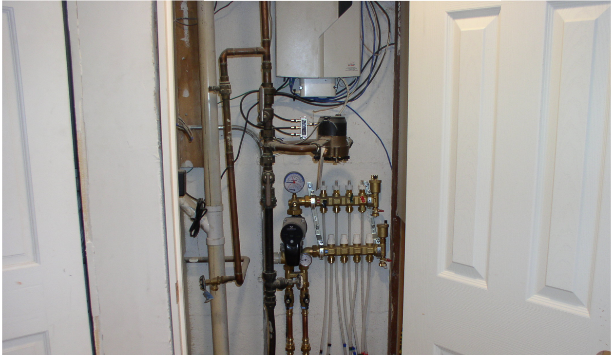
Zone 5 Basement Quick trac Caleffi 1725DAHE
