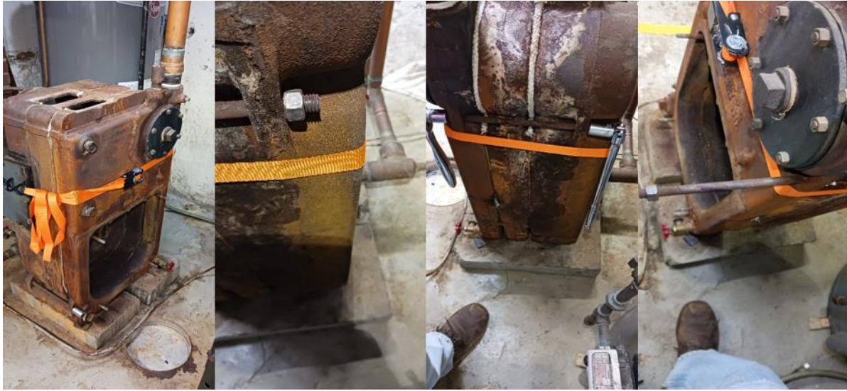
Figure 10 Tie Rod Removal Preparation Ratchet tie down was used to ensure the sections would stay together as the tie rods were removed. A \frac{3}{4} " socket on a \frac{1}{2} " breaker bar was used to loosen the nut on one end of the rod. The rod was in good condition so it was ultimately reused.
