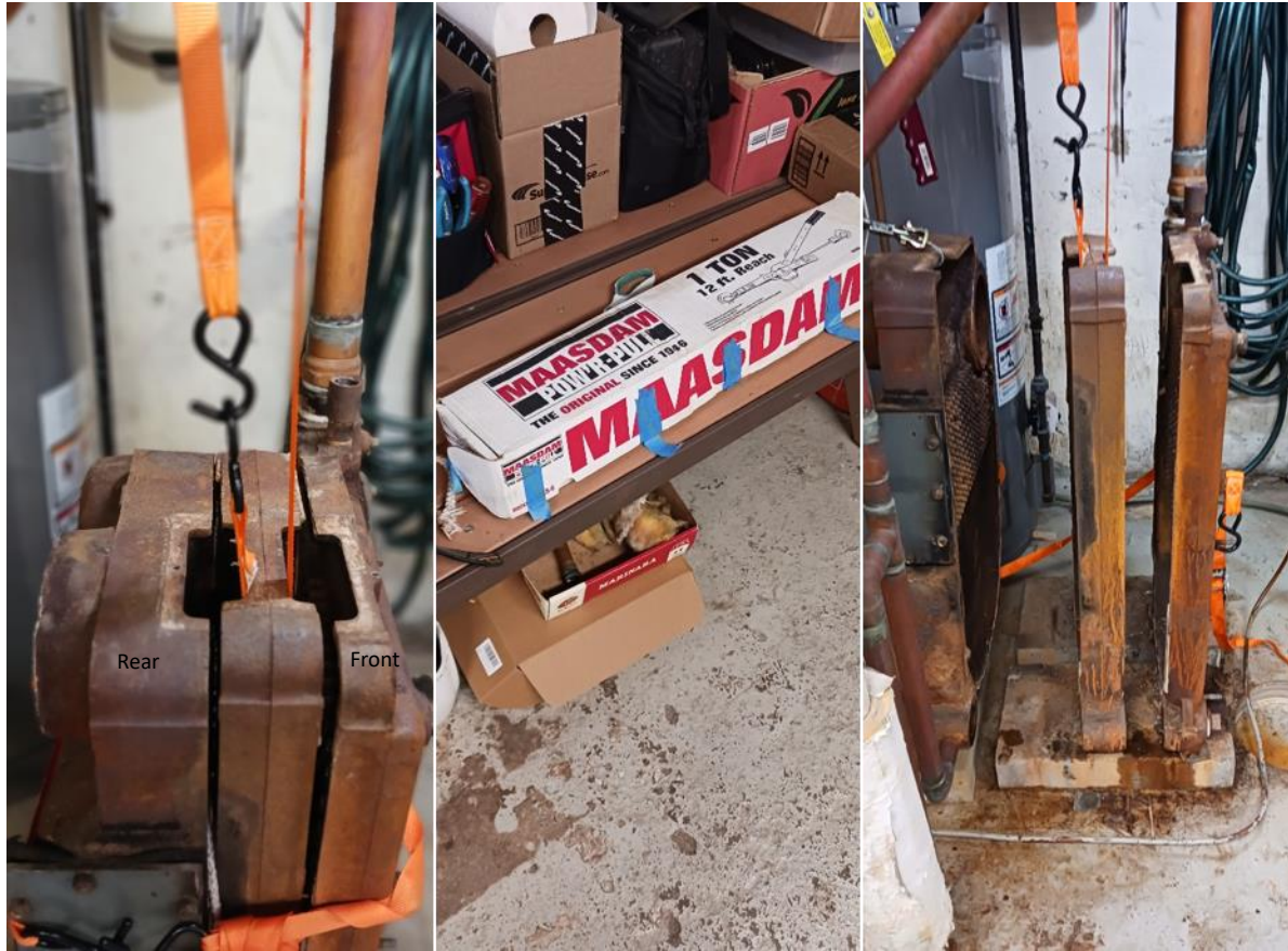
Figure 12 Rigging the middle section. Using a Maasdam come-along, the middle section was easily lifted out of place. It was heavy but could be lifted on to a nearby work bench by hand. Most of the rehabilitation and preparation was done on the middle section. With some care, the section was moved in and out of the assembly without using a come-along. The front section was still piped to the main header and remained in position throughout the rest of the rebuild.
