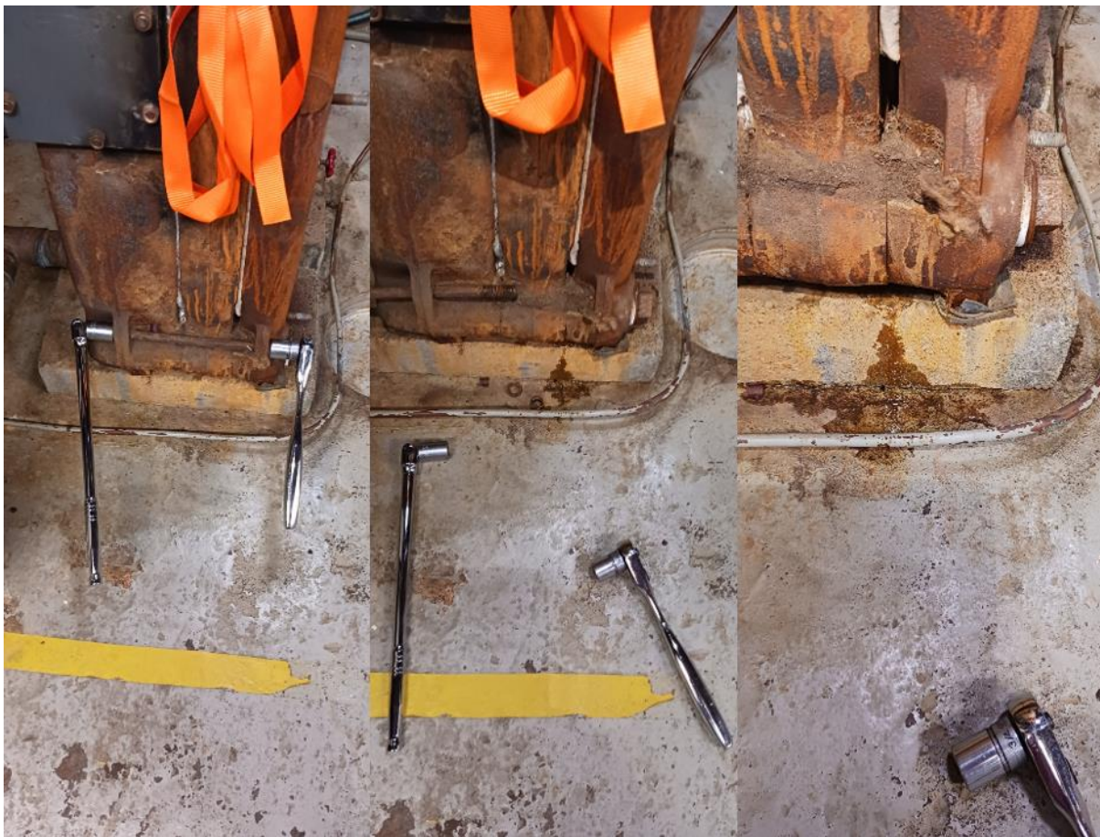
Figure 11 Lower waterside tie rod. Water immediately leaked out of the joint when the rod was loosened. Once the ratchet tie strap was loosened, the boiler sections separated without much more than by one hand.
