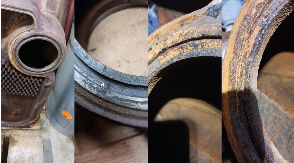
Figure 16 Restored section glands. The glands and faces were restored mostly with hand tools. The most effective tool for removing rust, scale, cement and cording was a ¼" wood chisel. It fit nicely into the gland and easily cut through any buildup. Pitting in the bottom of the gland was limited to a 20° arc and filled with JB Weld Steel epoxy. The restoration was better than represented in these photos. A very small void (a) was subsequently filled with another application of JB Weld. A steel file was used to dress across the surfaces. Most of the gland surfaces were very slightly damaged with only surface corrosion as seen in images 3 and 4. The planned sealing procedure was to use Permatex Red high temperature gasket material to seal all surfaces and create an adjunct gasket for the elastomer seals. The Permatex was painted on all mating surfaces with a thin layer using a small artist brush (stole from wife's art kit). The Permatex also provided a good slip layer during assembly to allow easy section alignment.
