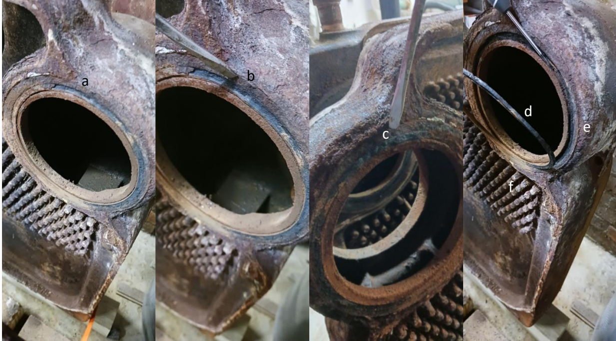
Figure 15 Steam side joints. The steam side joints were moderately compromised (a.) Both 6" elastomer seals had varying degrees of deterioration and lamination (b), causing corrosion of the glands but not on the opposing faces. A layer of the seal shown in (b) transferred to the opposing face (c). This evidence leads to the cause of failure where steam corroded the interface of the seal and gland and eventually eroded a path of escape. Corrosion of the glands was in a 20° arc and less than 0.020" deep at any point. The elastomer seals (d) were easily removed. They were still supple though not usable. It was a short path for steam to escape to the outside of the boiler (e) or to the inside (fireside) (f). The flue seal, part cement and rope were completely missing around the heater cavity. A fair amount of work was done to restore the groove that would seat the ¼" ceramic rope.
