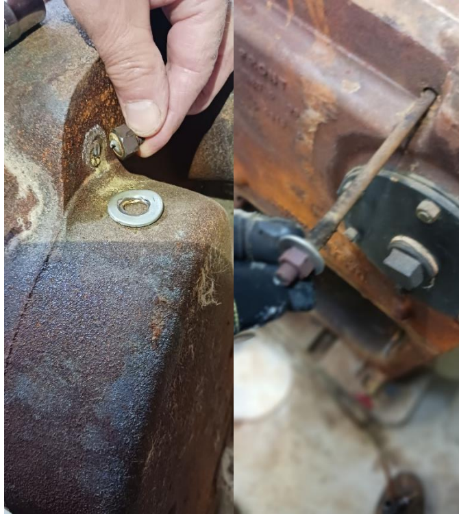
Figure 9 5/16" tie rod. This rod would have been exposed to steam causing the nut to seize onto the threads. Not much torque occurred before the rod sheared at the nut. There was no split-lock washer on the tie rod.
