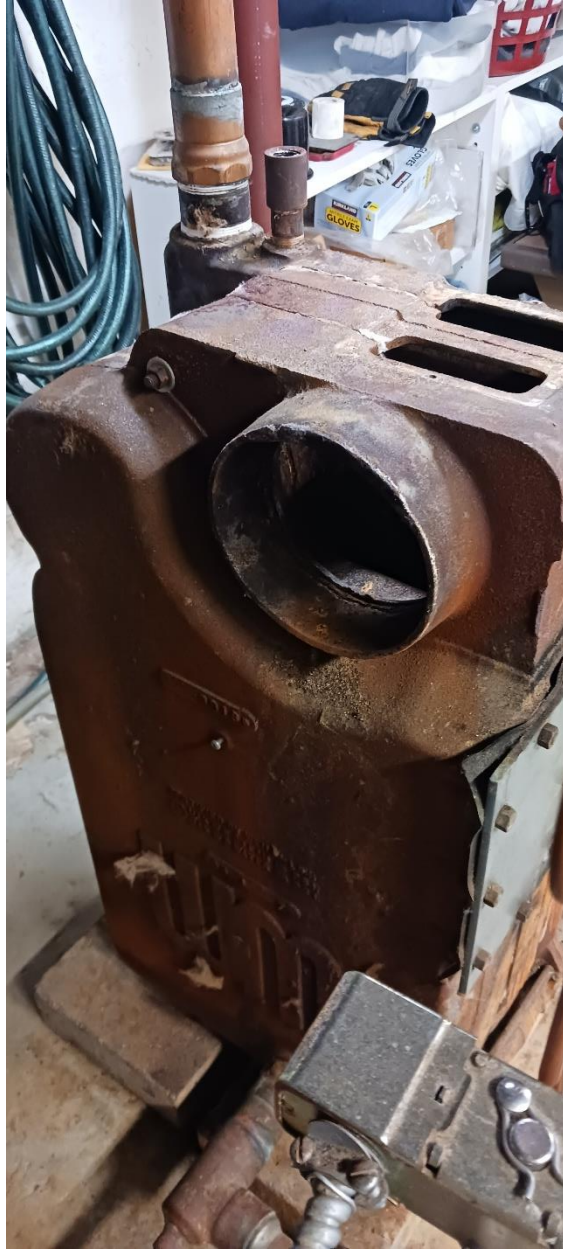
Figure 7 Boiler rear section. The rear section was isolated from the existing piping by cutting a 1-1/4" copper condensate return pipe leading to the 2" main boiler port. This rear section was too big and heavy to remove from its location on the pillow block. The best that could be done to facilitate movement of the section was a come-a-long secured to the ceiling joists above the boiler. At times, the section was tilted backward to rest on the bottom blow-down valve. Solenoid for automatic water fill valve is shown (lower right.)
