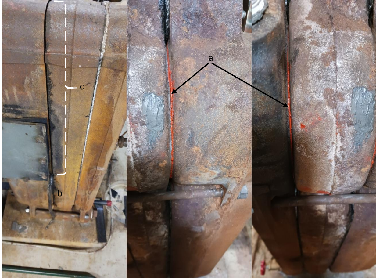
Figure 17 Reassembled boiler sections. A small amount of Permatex gasket material squeezed out of the 6" upper joints(a). Tie rods were torqued to 50 ft-lb for the 1/2" rod (as per Weil-McLain technical support) and 25 ft-lb for the 3/8" rod (as per calculated yield for carbon steel.) Sections were allowed to rest for 24 hours then re-torqued with some tightening. After another 24-hour relaxation, no further tightening occurred at torque values. After three practice dry assemblies, it was learned that the ceramic rope was impeding the 6" rear/middle sections from mating. A length of rope (b) was eliminated from the assembly to allow the sections to mate. The gap (c) was later filled Rutland 2000°F furnace cement. Both joints were then covered with cement (not shown.) Boiler was hydrostatically tested to 4 psi for 24 hours with no leaks. Boiler was tested to 2 psi steam pressure with no leaks (water or smoke). Boiler cycled several times and has been at rest for 5 days without leaks.
