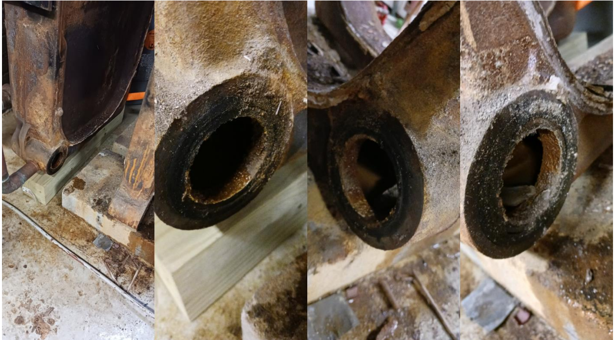
Figure 13 Waterside joints. The seal glands and opposing faces of the water section joints were found to be in very good condition. Though they look rough in these photographs, they cleaned up easily to almost new condition. The 3" elastomer are still emplaced in their glands.
