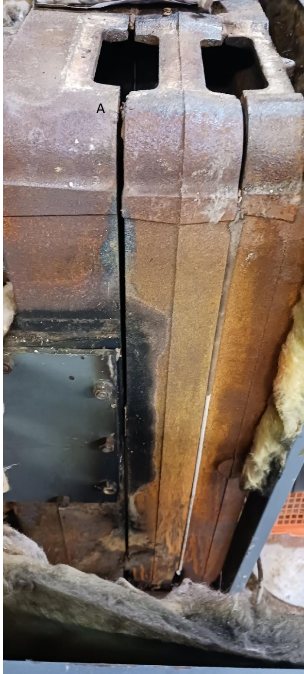
Figure 2 Fireside joint failure. Long region of inter-section sealant allowed combustion smoke to escape the combustion/flue passage and into the room. Smoke residue is apparent on middle boiler section and adjacent Cover Plate for Heater Opening (Rectangular.) Middle boiler section (A) is misaligned with the front and back sections. Bead of sealant between front and middle section remains mostly intact. This condition started very early in the life of the boiler but was only noticed on a poor ignition instance. There was only ever a puff of smoke that escaped at ignition and a nearby smoke detector about the boiler never detected smoke.
