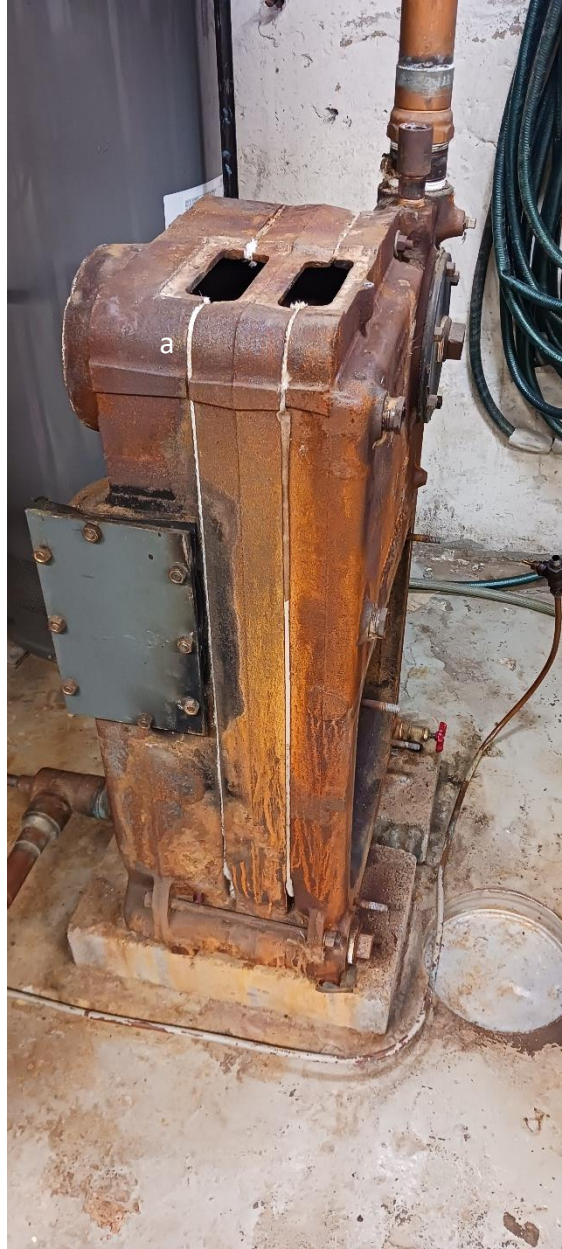
Figure 6 Boiler side view. \frac{1}{4} " ceramic rope (measured closer to \frac{3}{8} ") was packed into gap (a) between the rear and middle sections. By stretching the rope and forcing it with a putty knife, the rope was neatly emplaced to seal off combustion gases. This step was taken to seal off escaping flue gases before the steam leak on the opposite side was discovered.
