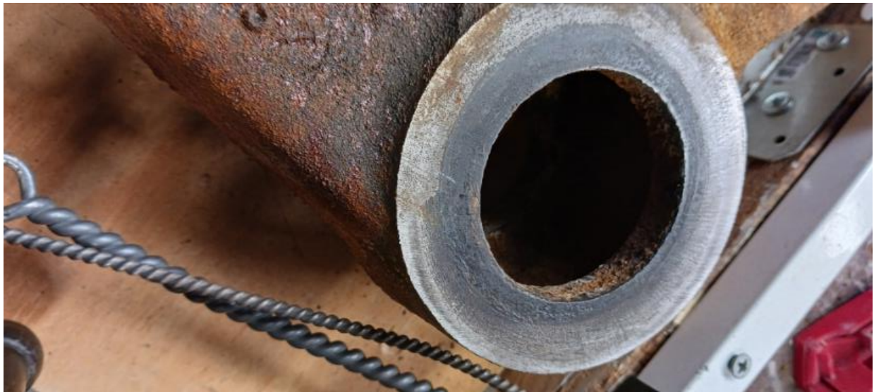
Figure 14 Restored waterside-joint face. The faces of the section joint were all very near perfect. A file and emery cloth were used to remove and deposits and clean the surfaces. A minor amount of corrosion was located to the inside diameter of the elastomer seal, otherwise, the surface was intact.
