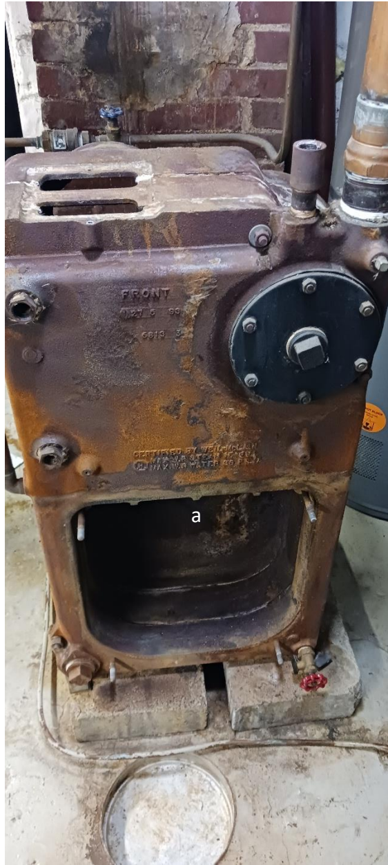
Figure 5 Boiler Front. The fire box was significantly deteriorated (not shown). Evidence of steam or condensate infiltration (a.) The boiler was deemed no longer usable and was taken out of service.
