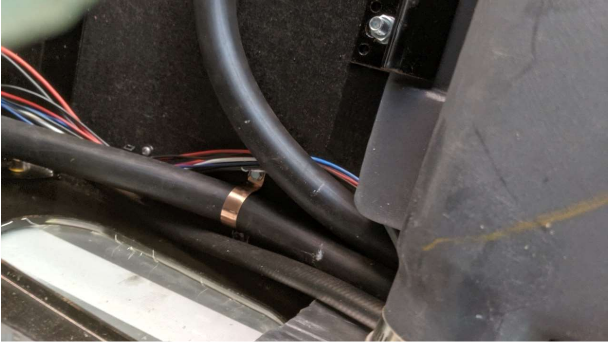
Some pictures of the pipe runs:
